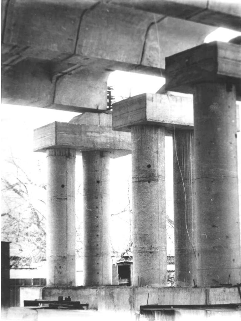
Figure 4.25. Operation of the piers compressed using the During-tensioning method for the bridge supports over the Dnieper River in Kamianske
