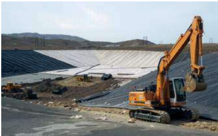
Fig. 7. Creation of an anti-filtration screen using geotextile material during the construction of a landfill for waste storage
