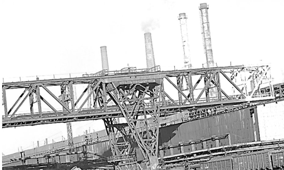
Fig. 1. Appearance load-bearing structure of the reloader (cantilever section).
