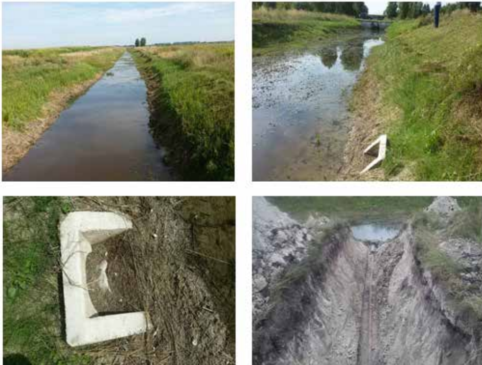
Figure 8. Condition of the open channel MC-28 and the outlet of the closed horizontal drainage DC-1 in the Melnytska drainage system
