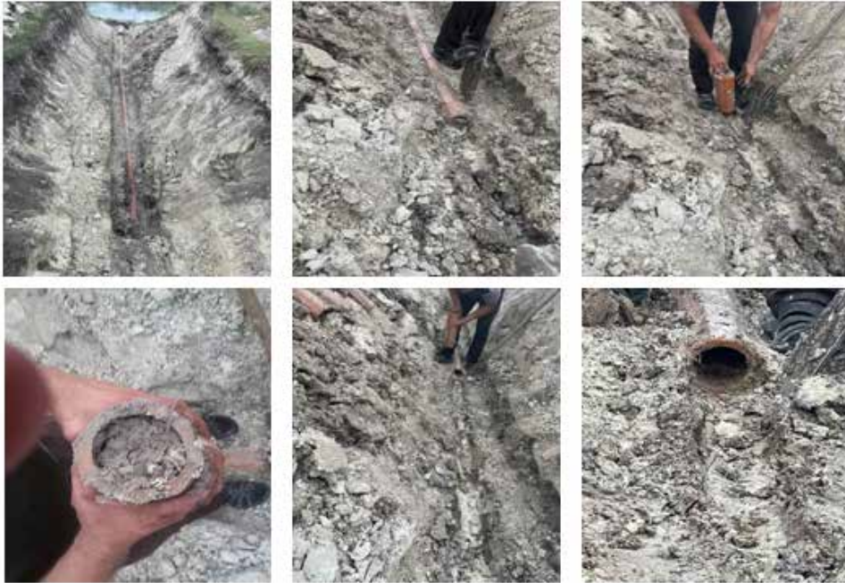
Figure 9. Excavations of closed horizontal tile drainage with ceramic pipes on collector DC-1
