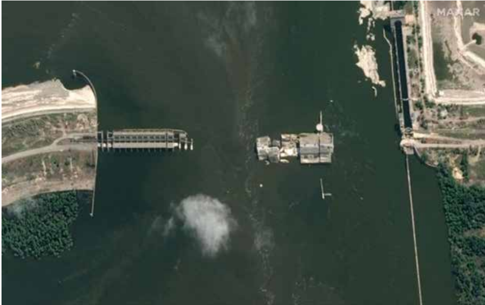
Figure 1. The current state of the Kakhovka Dam after the explosion
